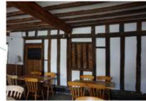
Southern room on the ground floor with early 16 th Century timber frame and later alterations
